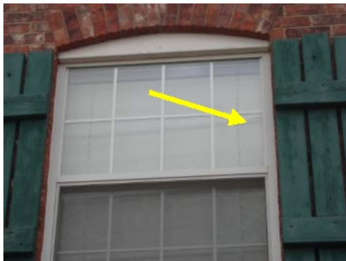
Cracked window in upstairs bedroom
