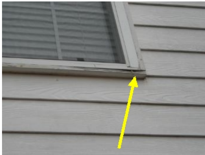
Rotting window trim
