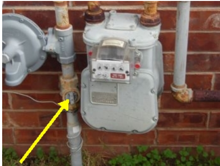
Main gas shut off
